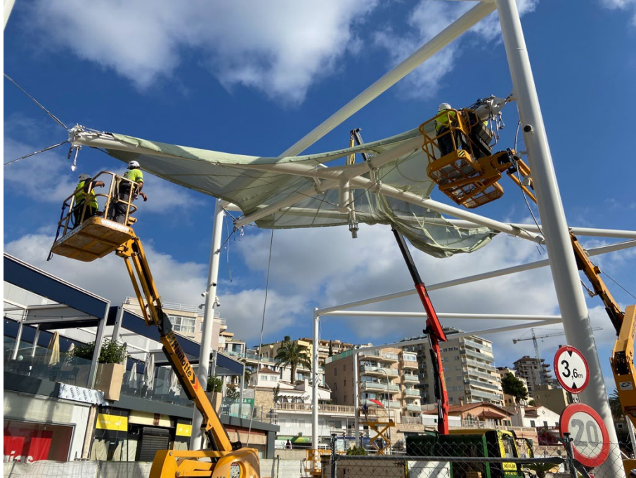
Figure 19 Assembly of one of the conoids using small cranes and cherry pickers
