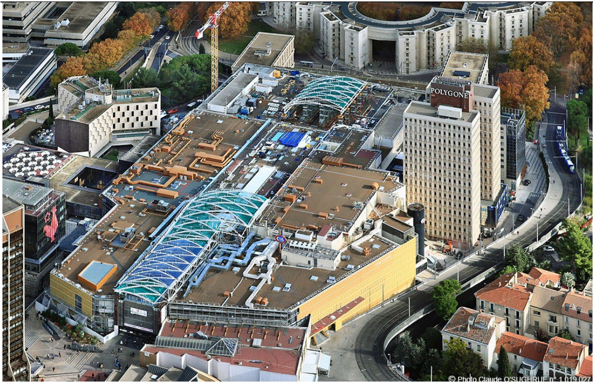
Figure 5: Blocks n°1 and n°2 already moved to their final position, and block n°3 being assembled on the working platform.
