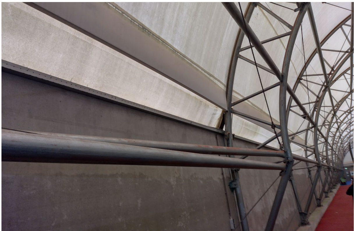
Figure 3: inside picture of the tennis court (the orange gravel dust everywhere discloses it is a tennis court)
