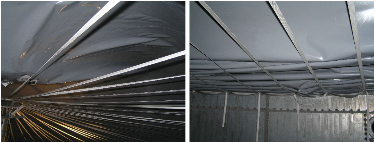
Figure 3: Placing the gas membrane on the belt system during emptying, Lowering the pole cap (right), radial folding form the tank edge (right).
