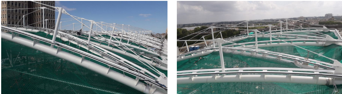
Figure 7: Assembly of aluminium frames on a propped metal structure before deformation under its own weight.
